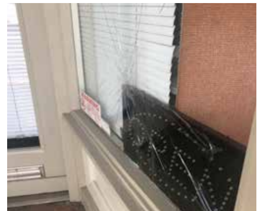
Broken window on Nuuanu Ave.
