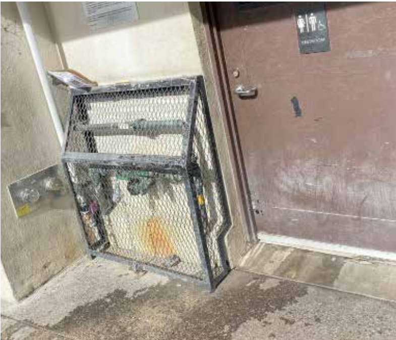
Waste water from public toilet flows to sidewalk
