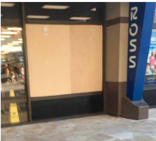
Window broken at Ross, Fort Street Mall
