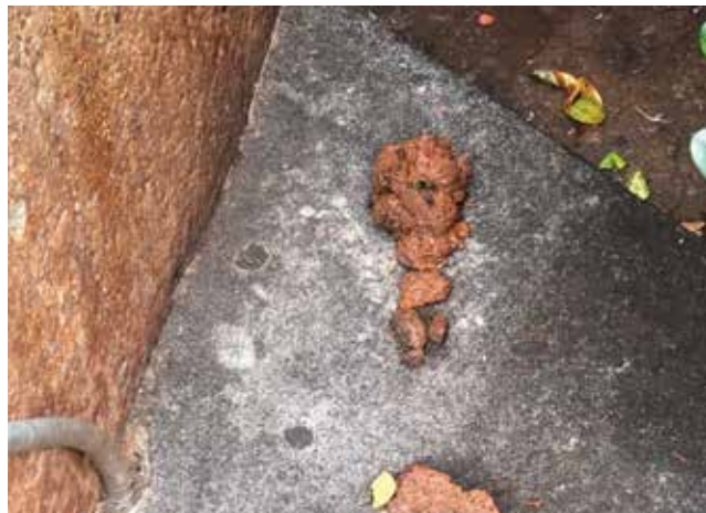
Feces on walkway
