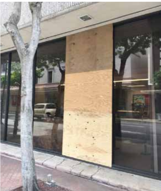
5th broken window in a year at HNB, King St.
